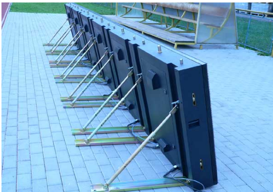
Stadium Cabinet Structure
