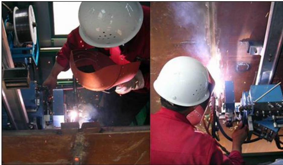
Inside the EGW frame
